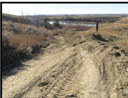
Water diversion earthwork completed by the McKenzie County Roads Department adjacent to the Cartwright Train Tunnel.
